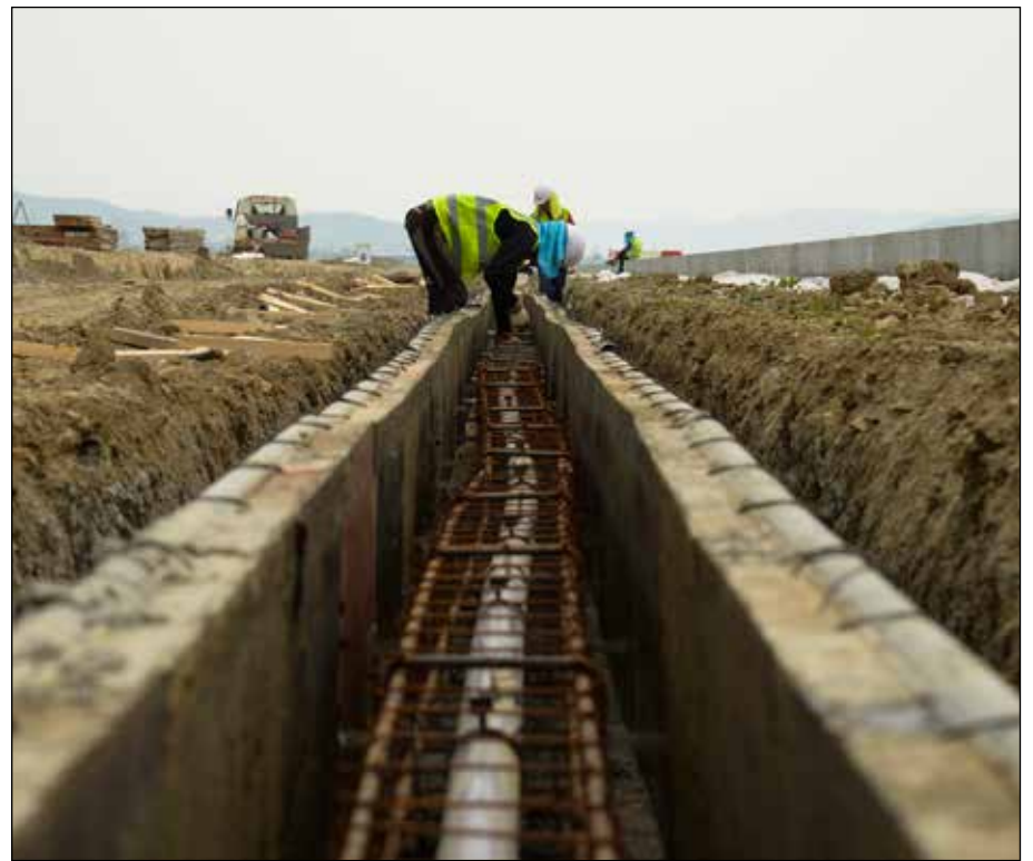
Republic of Korean contractors work on the second runway April 28, 2015, at Osan Air Base, Republic of Korea. The runway is being designed to buttress Team Osan's operations and alleviate stress on the base's single runway. (U.S. Air Force photo by Staff Sgt. Jake Barreiro)
