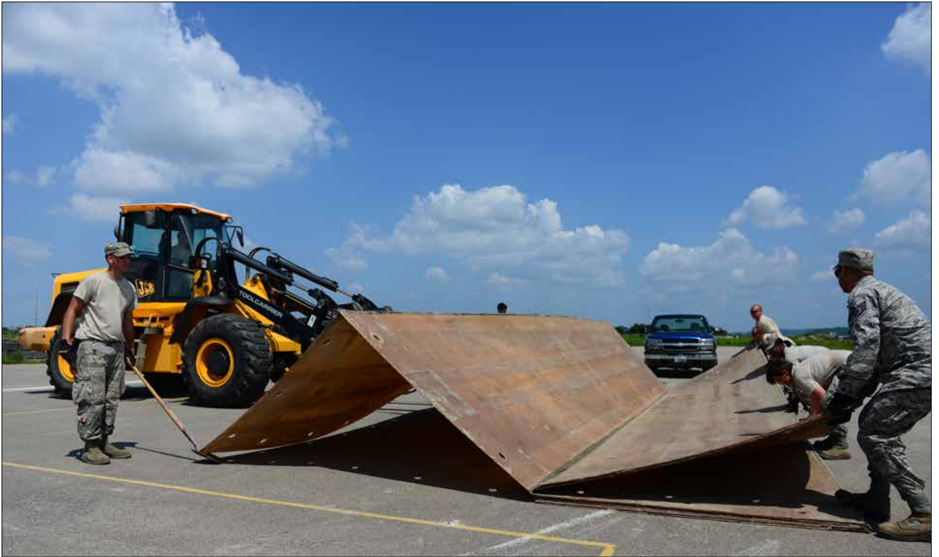
Airmen from the 51st Civil Engineer Squadron structures shop unfold a large rapid-runway repair fiberglass mat as part of airfield damage-repair drills at Osan Air Base, Republic of Korea, Aug. 18, 2015. Known as the catch-all career field, structures Airmen have a job that can vary from the indoors, outdoors, homes, office buildings, the flightline and everywhere in between. (U.S. Air Force photos by Staff Sgt. Amber Grimm)
