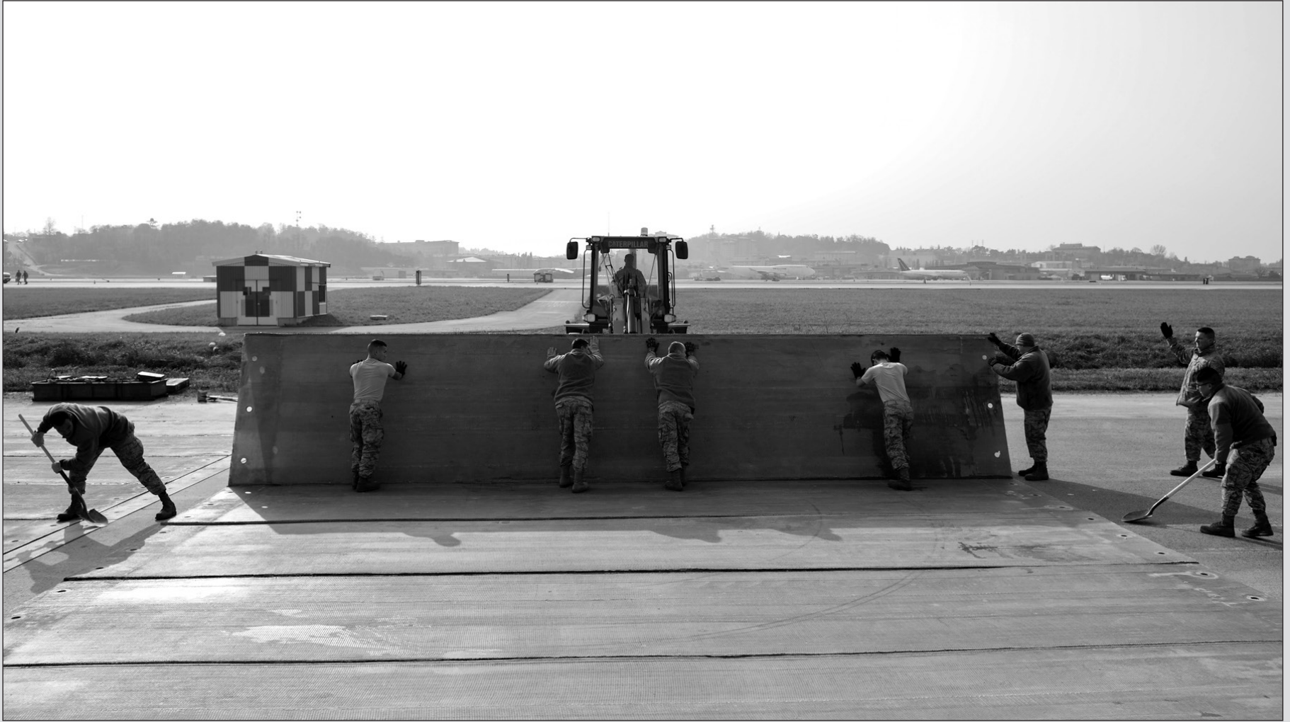
Airmen from the 51st Civil Engineer Squadron structures flight consolidate a folded fiberglass matt during Prime Beef Day at Osan Air Base, Republic of Korea, Nov. 17, 2016. Folded fiberglass matts are used to help reinforce damaged runways during contingency operations, with the ability to withstand the weight of a landing aircraft without fracturing. (U.S. Air Force photo by Senior Airman Victor J. Caputo)
