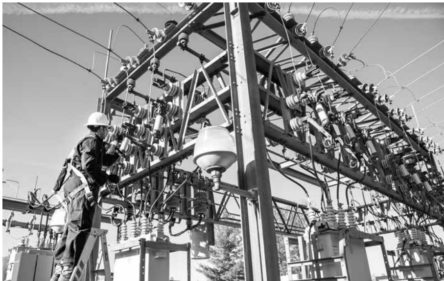
Staff Sgt. Manoj Williams, 375th Civil Engineer Squadron electrical systems craftsman, greases framework knife blades and tightens loose conductor connections April 9, 2016, at Scott Air Force Base, Ill. The base required a scheduled power outage to repair critical high-voltage electrical components. (U.S. Air Force photo by Airman Daniel Garcia)
