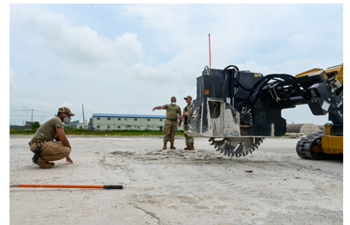
Airmen from the 8th Civil Engineer Squadron ensure a pavement saw is in the proper position during exercise Beverly Sentinel 25-3 at Kunsan Air Base, Republic of Korea, Aug. 6, 2025. The 8th CES practiced Rapid Airfield Damage Repair (RA/DR) to ensure they maintain the ability to quickly restore damaged airfields after attacks, enabling flight operations to continue. (U.S. Air Force photo by Senior Airman Karissa Dick) ▲
