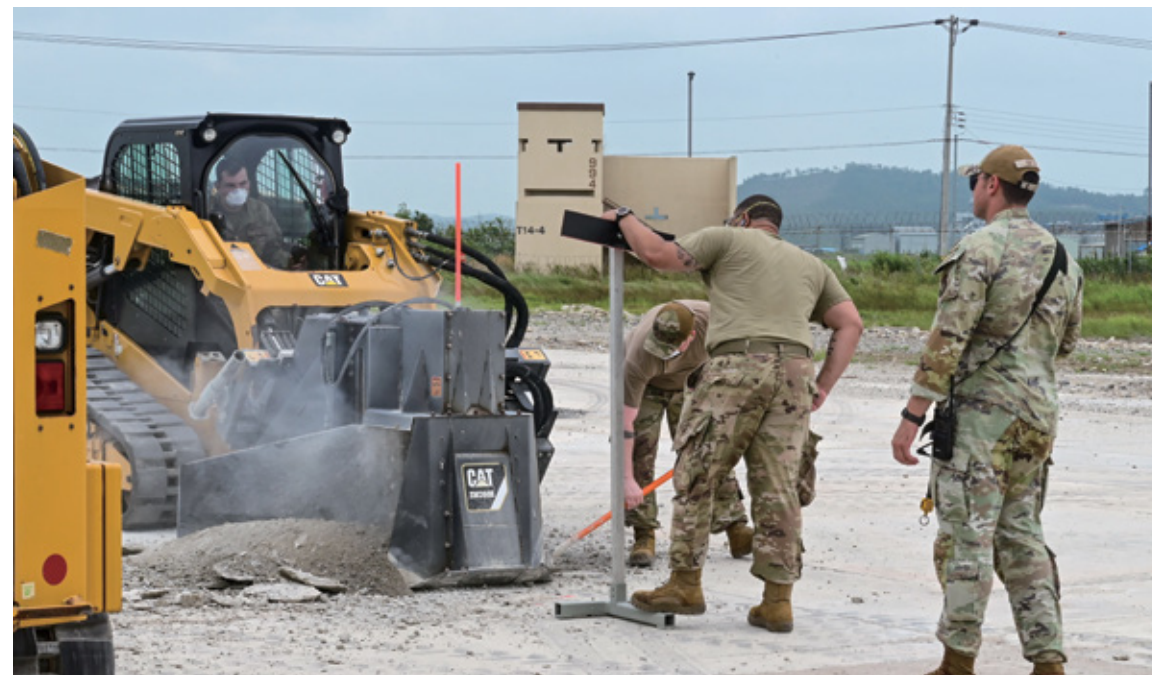
Airmen from the 8th Civil Engineer Squadron transfer water into a cement mixing truck during exercise Beverly Sentinel 25-3 at Kunsan Air Base, Republic of Korea, Aug. 6, 2025. The 8th CES practiced Rapid Airfield Damage Repair (RA/DR) to ensure they maintain the ability to quickly restore damaged airfields after attacks, enabling flight operations to continue. ▶
