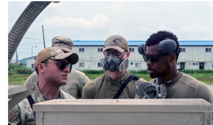
U.S. Air Force Staff Sgt. Luis Romano, 8th Civil Engineer Squadron heating, ventilation and air conditioning spall team member, smooths a concrete patch over a hole during exercise Beverly Sentinel 25-3 at Kunsan Air Base, Republic of Korea, Aug. 6, 2025. The hole was created on an area of the flightline where the Red Devils practice Rapid Airfield Damage Repair (RA/DR). ◀
