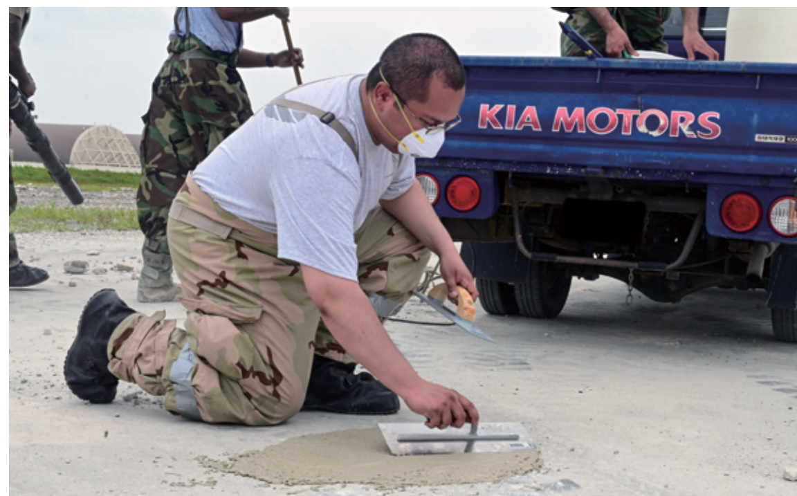
Airmen from the 8th Civil Engineer Squadron move debris away from a pavement saw during exercise Beverly Sentinel 25-3 at Kunsan Air Base, Republic of Korea, Aug. 6, 2025. The saw was used to cut out a measured section of the flightline where the Red Devils practiced repairing airfield damage. ▼
