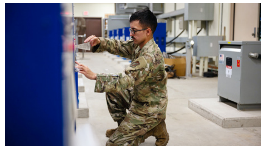
U.S. Air Force Staff Sgt. Jose Medina, 51st Civil Engineer Squadron electrical systems craftsman, troubleshoots different current intensities at Osan Air Base, Republic of Korea, Sept. 3, 2025. The constant current regulator is responsible for sending electricity to all parts of the flightline, keeping signs and lights lit everyday for flightline operations. ▲
